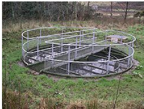
Figure 5. Secondary Sedimentation tank at a rural treatment plant.
